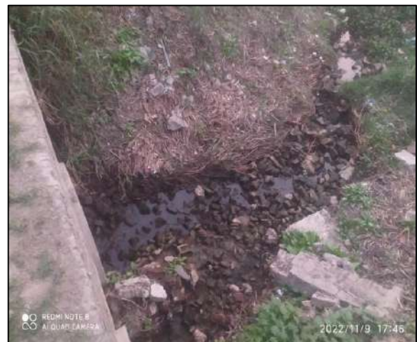
Figure 74 Kinauni Drain confluence with River Hindon
